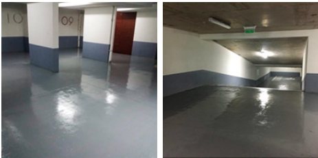
Dust sealer and wear protector application for cellars (Considers supply of materials and specialized labor)
