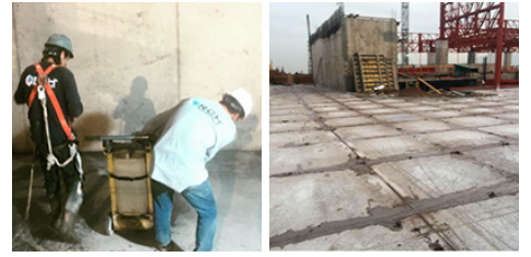
Expansion and insulation cuts with water cooling disc (Recommended for under-roof or thick foundations)
