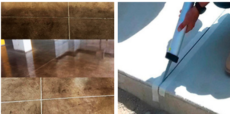
Seal of expansion joints, insulation and construction (Considers supply of materials and specialized labor)
