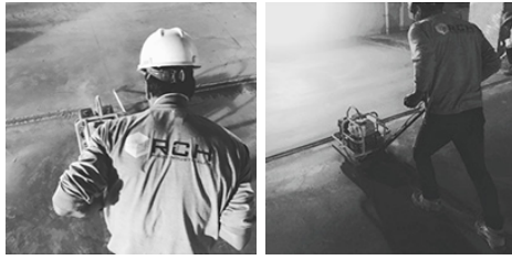
Expansion and isolation cuts with Soff-Cut system (Recommended for low thickness or early maturing foundations)
